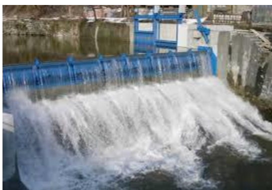
Figure 1 A mini hydro power plant operated by an IPP in Zimbabwe
