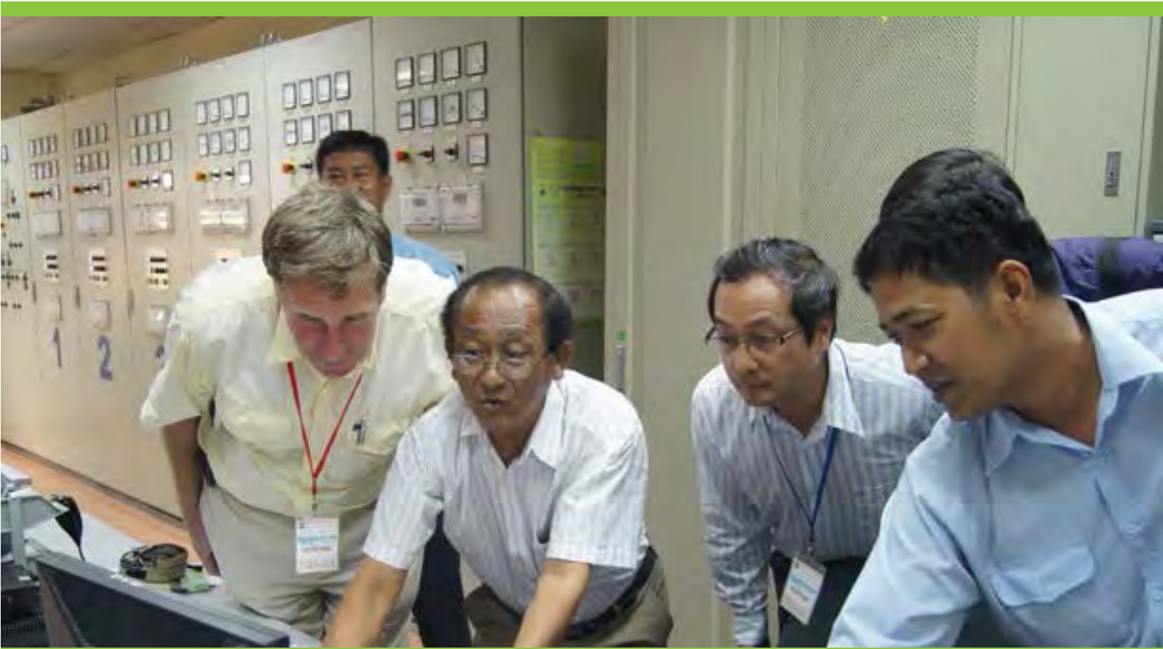
Power generation controls being demonstrated to the SEA team at an oil-fired power station, Phnom Penh, Cambodia
